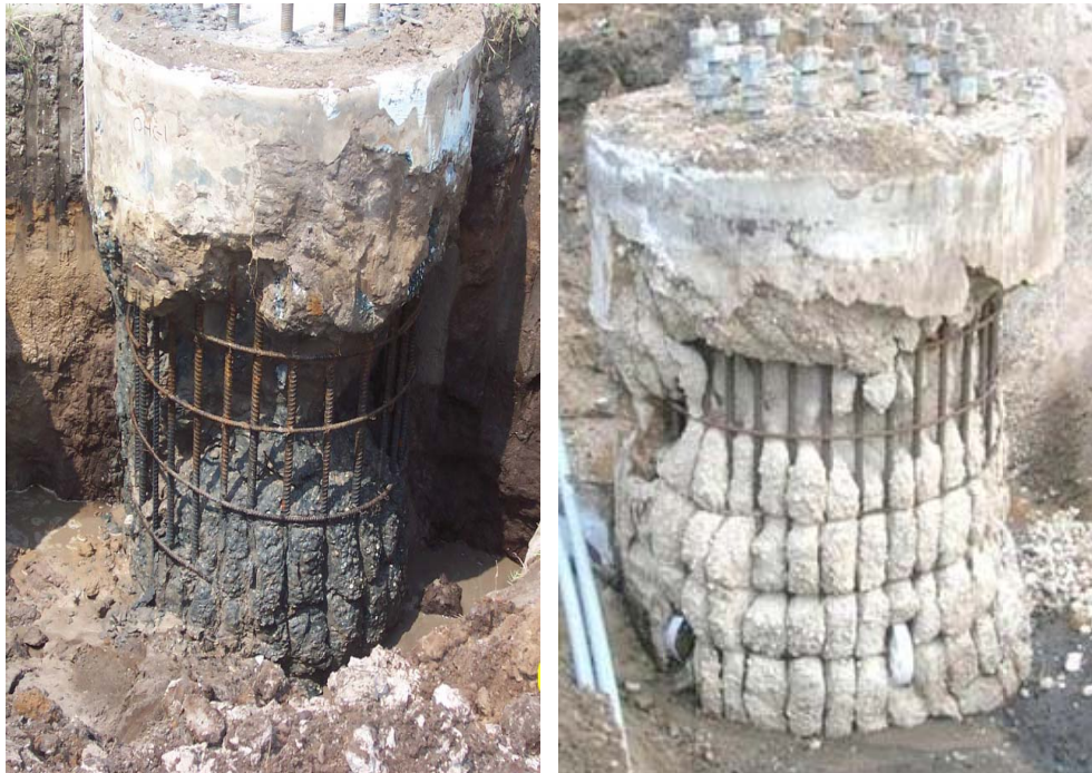
Figure 1.4 Underground flaws in drilled shafts that required excavation to identify.
