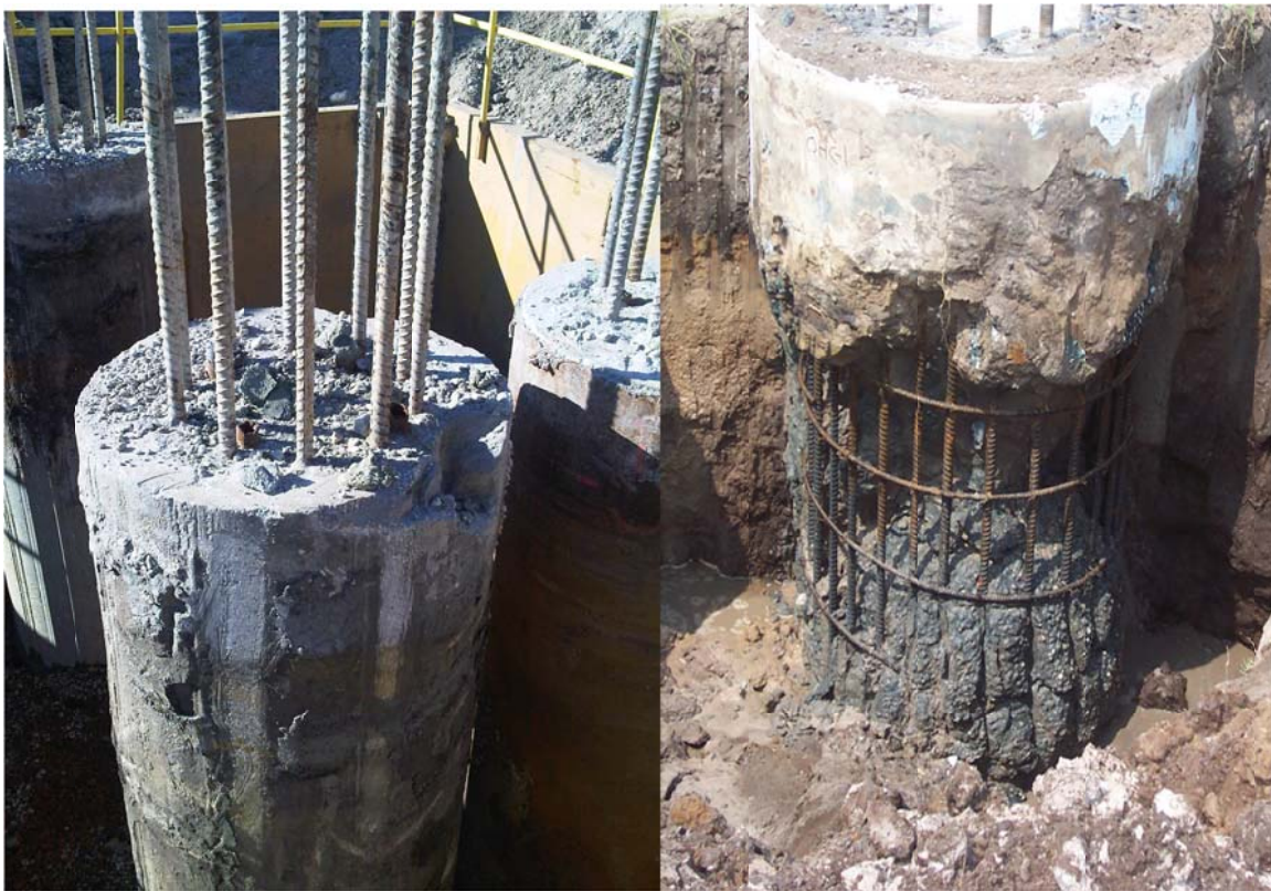
Figure 3.2 Visually intact shaft (left); visually deficient shaft (right).
